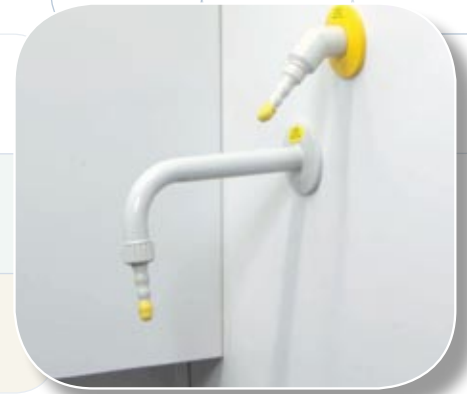
Service fixture outlet is mounted on the cabinet.
